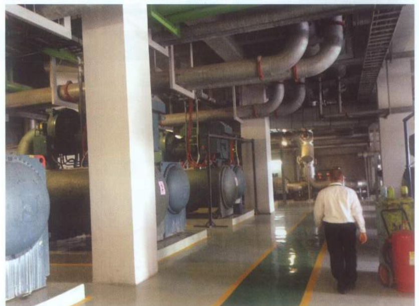
CIRCULATION PATHWAY CLEARLY MARKED IN PLANT ROOMS
